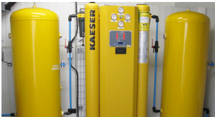
Top: Three PCI Oxygen Generators are installed in the containerized steel frame gas handling building. Above left: Desiccant drier system and right, two Kaeser air compressors
