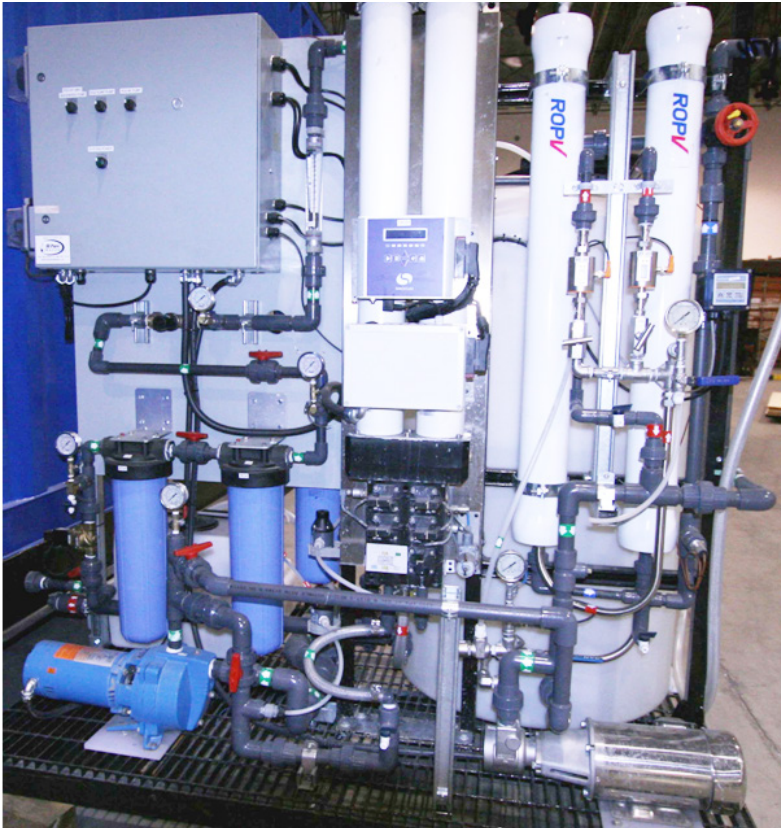
A pilot plant identified appropriate membranes capable of treating the difficult mine wastewater
